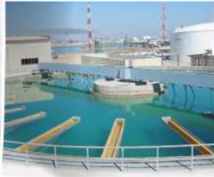
Industrial water treatment
